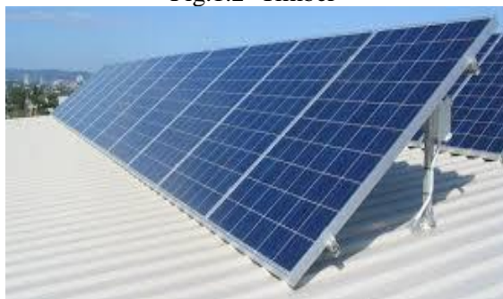
Fig.2:- Solar Panel System
